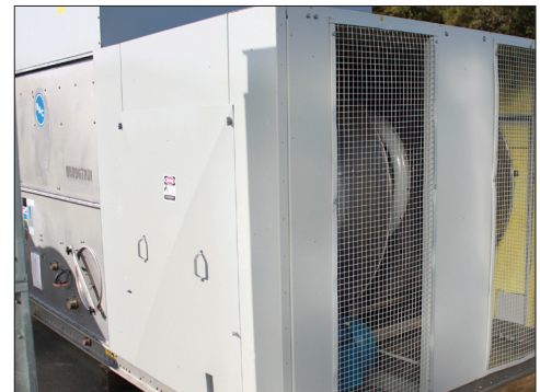
Intake Sound Attenuation
