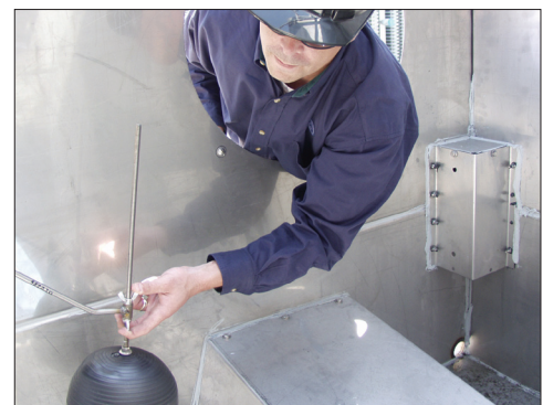
Standard Mechanical Water Level Control
