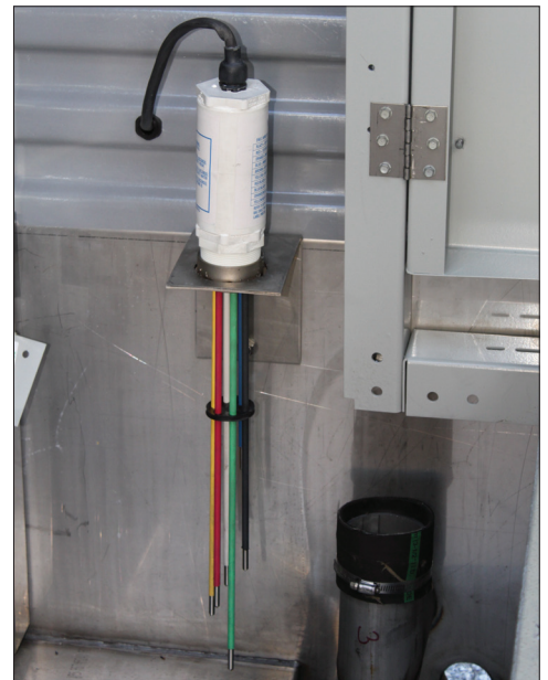
Electric Water Level Control
