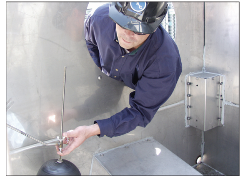
The Water Level Control is Easily Reached From the Access Door
