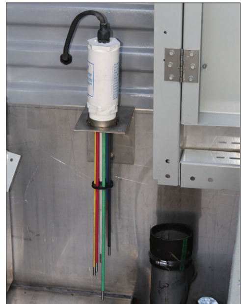
Electric Water Level Control
