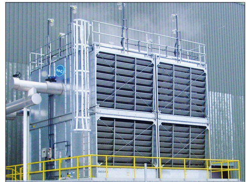
External Ladder, Safety Cage, and Handrail
