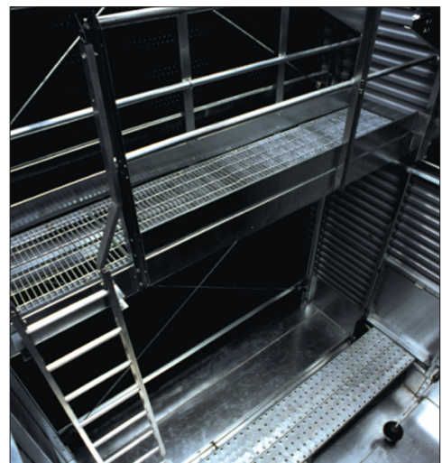
Internal Ladder, Service Platform, and Walkway
