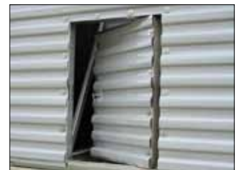
Large Access Door
