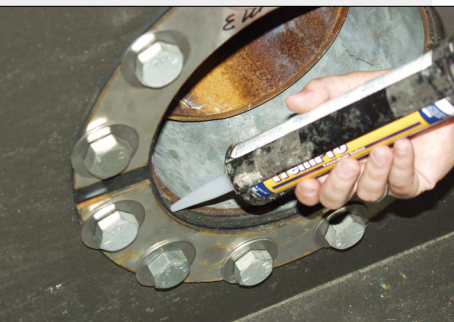
Figure 13. Caulk Exposed Galvanized Steel
