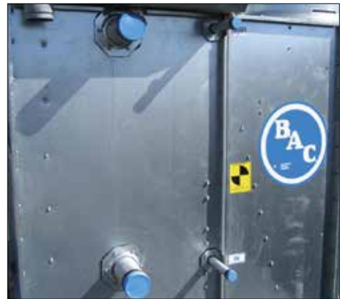
Multiple Circuit Coil
