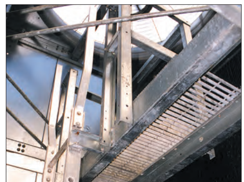
Internal Service Platform and Internal Ladder
