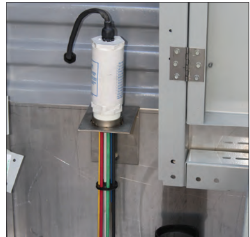
Electric Water Level Control
