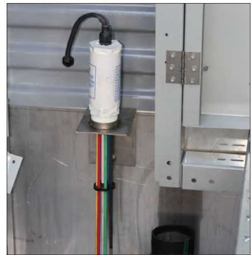
Electric Water Level Control (EWLC)
