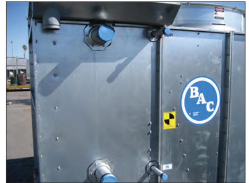
Multiple Circuit Coil
