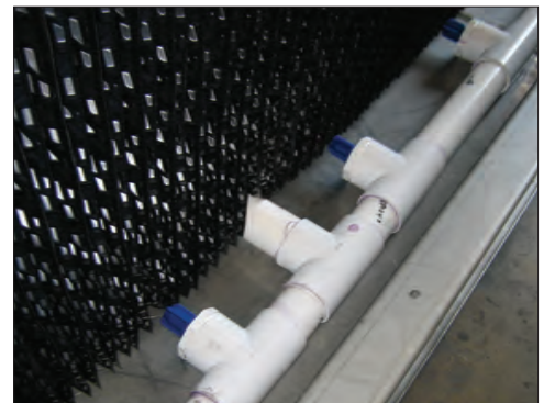
Basin Sweeper Piping
