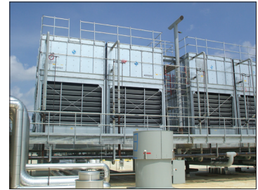
Multi-Cell FXV3 Installation Showing Simplified Piping
