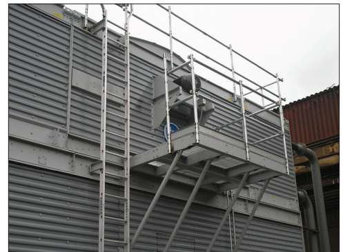
External Motor Platform
