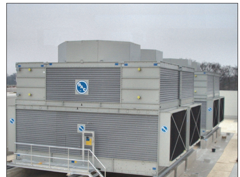
Intake and Discharge Sound Attenuation
