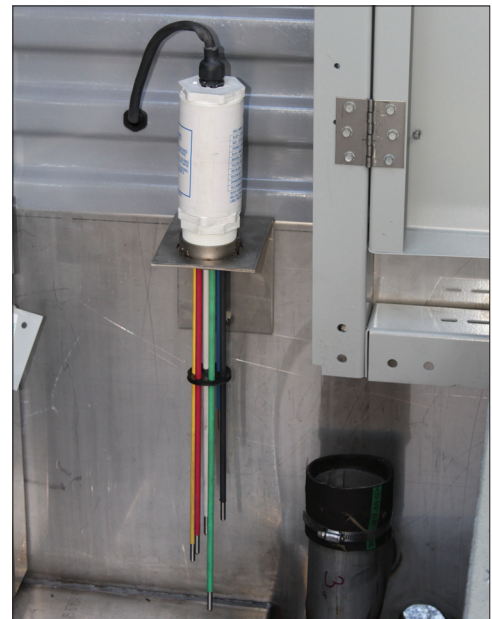
Electric Water Level Control
