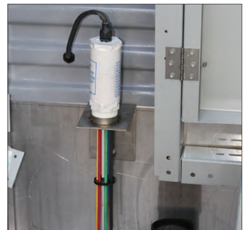
Electric Water Level Control
