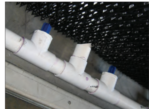
Basin Sweeper Piping
